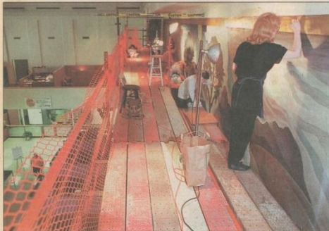
Joyce Hill Stoner works on scaffolding to restore a 66-year-old N.C. Wyeth mural at the Wilmington Savings Fund Society building in Wilmington. She says the difference in colors is like "night and day."
